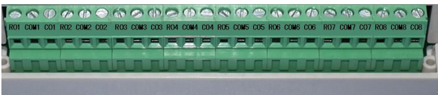
Relay controller output terminal block
